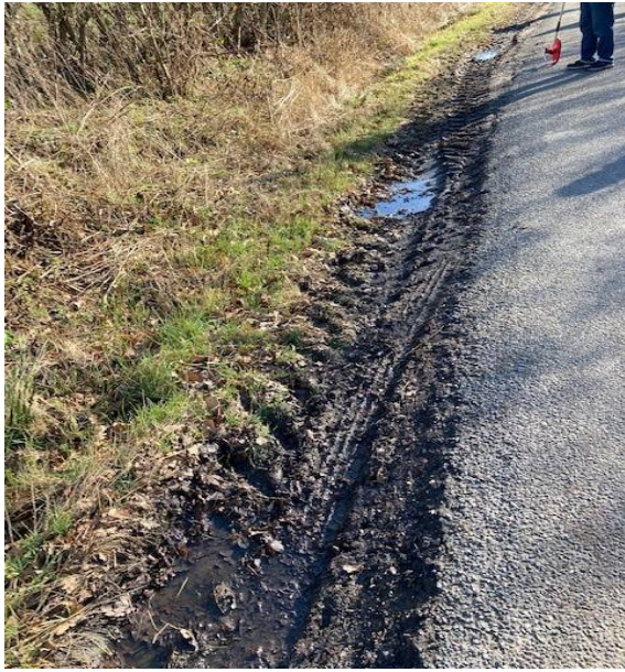
50. To show extensive damage to land and road edge. No safe haven, no passing places and no refuge point for non-vehicle road users
