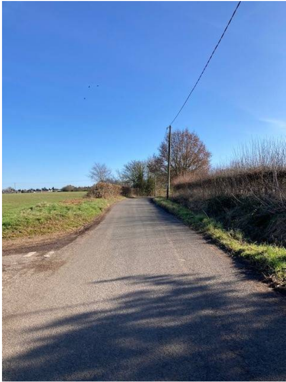
39. Junction of Kelvedon Road and New Road. No signs in New Road. Road is bordered by deep ditches
