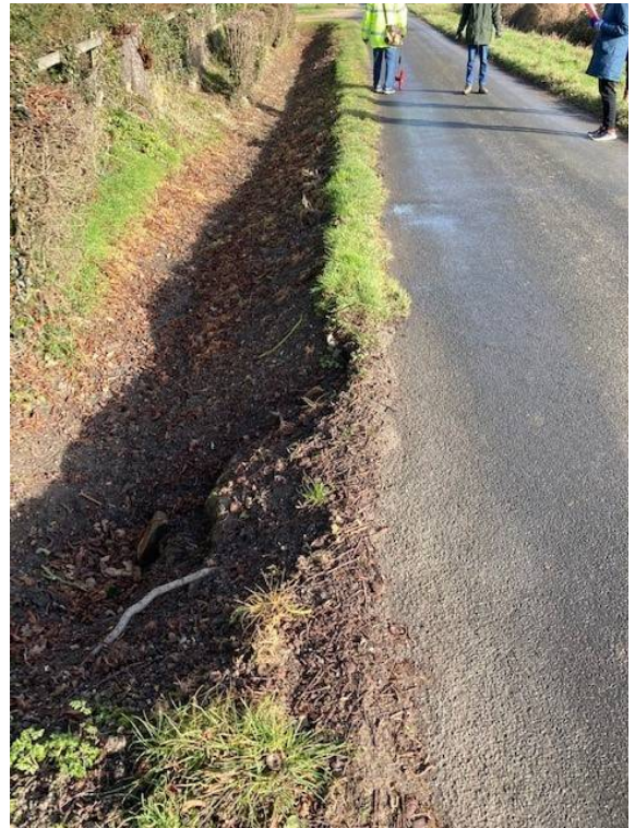
47. To show deep ditches within 20cm of road edge. No signs, no warning
