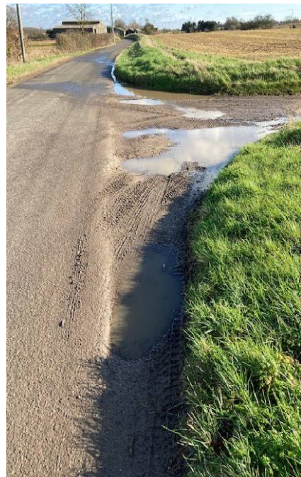
6. Extensive damage and destruction to road edge
