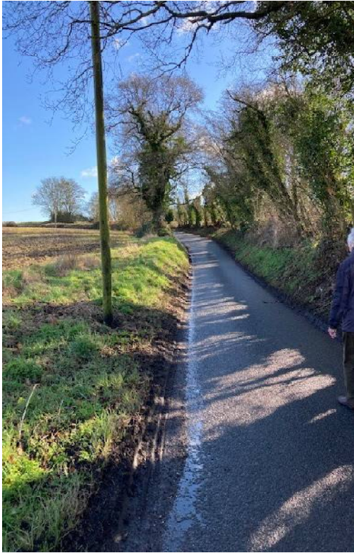
3. Damage to verges and unsighted road
