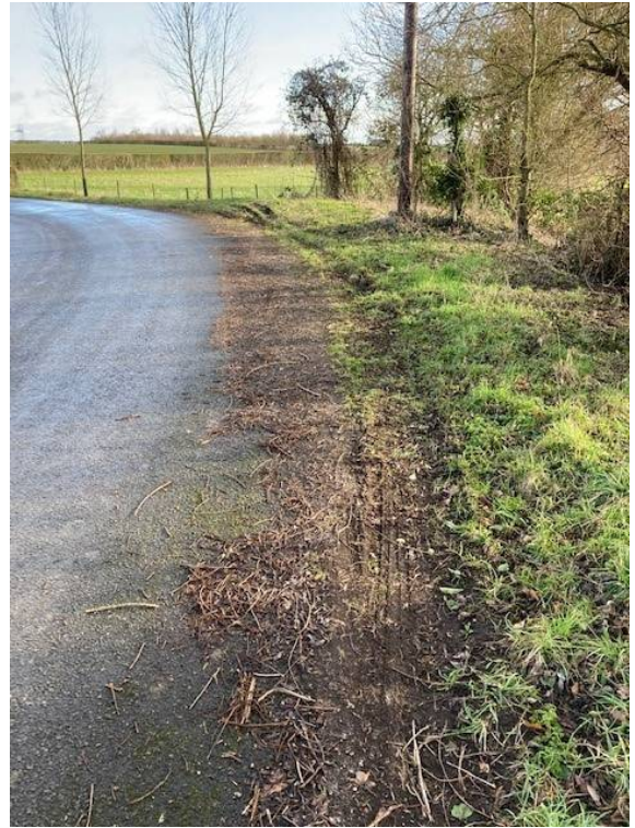
49. To show massive damage caused by existing traffic. No safe havens no pavement and no refuge
