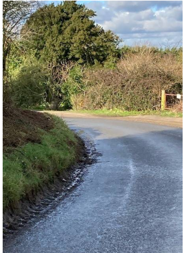
12. Road damage to high verges and blind bend
