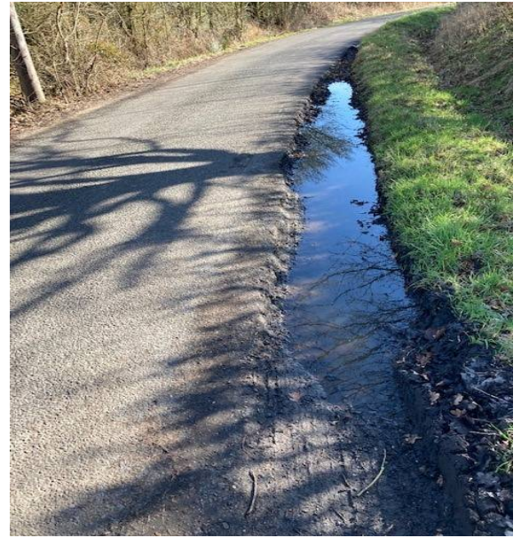
51. Showing extensive road deterioration and damage, no signage warning of school and no safe haven for pedestrians and children
