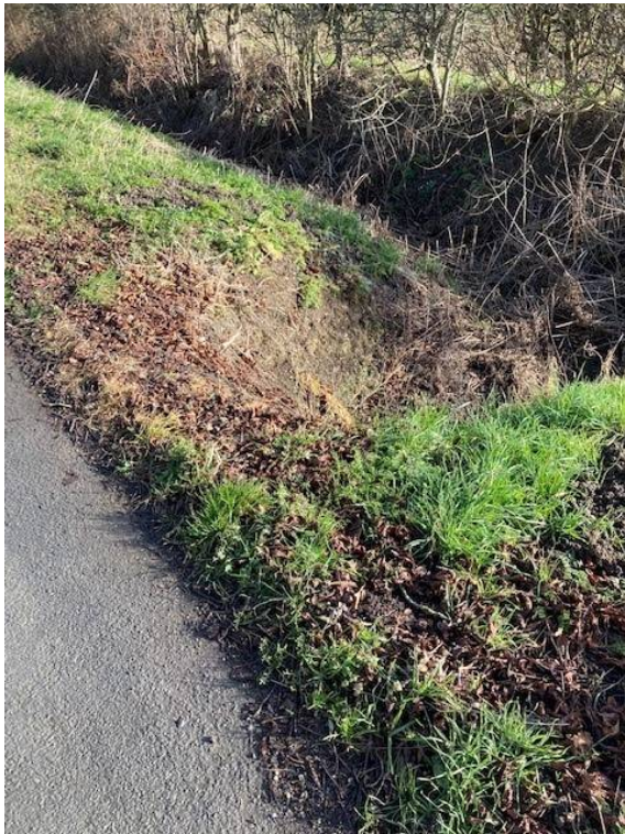
46. To show hidden deep drainage ditch, and road edge erosion
