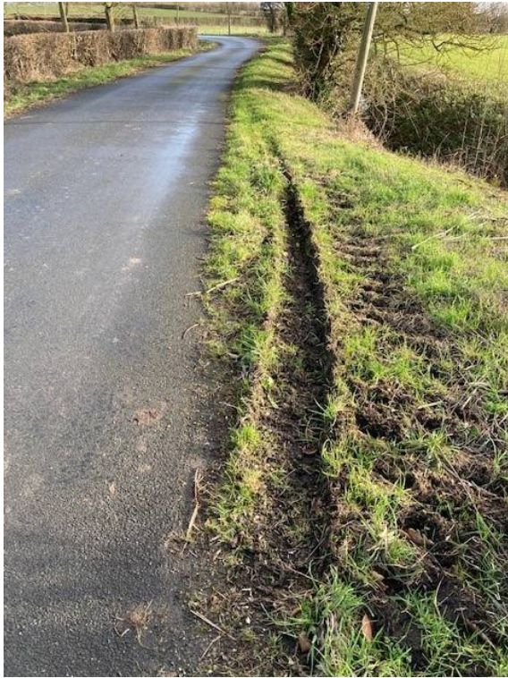
48. To show extensive damage to verges and edges caused as traffic forces a passing place
