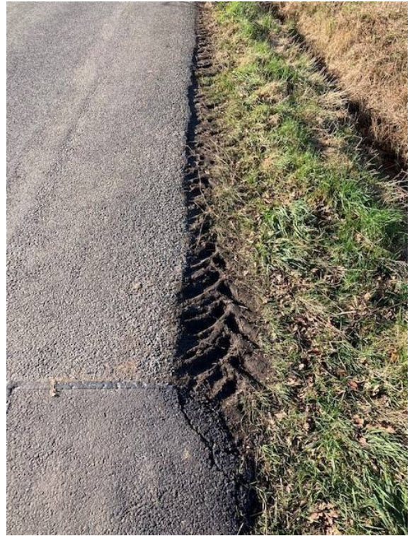
36. To show extensive damage to land as traffic forces a passing place
