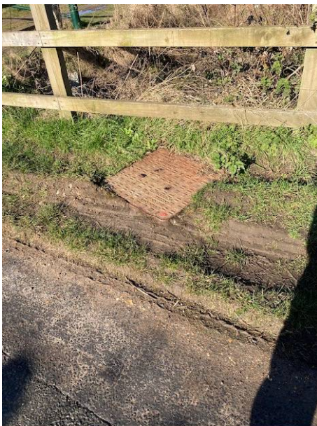
66. Raised manhole, within 25cm of road edge, already substantially damaged by existing traffic
